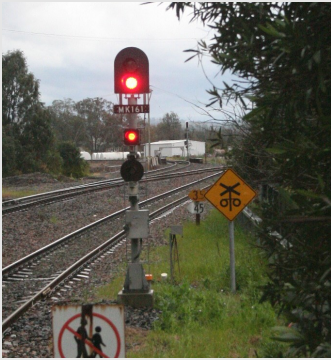
MGB International have designed several Microlok and Relay interlockings for ARTC North Coast Corridor
